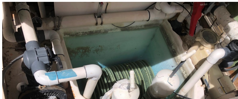
Pool circulating pump on right. Pool filters on lower foreground.
