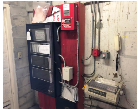
Fire Alarm Control Panel
