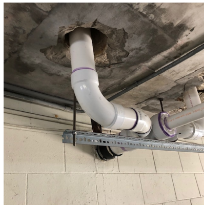
Concrete spalling (pops)
