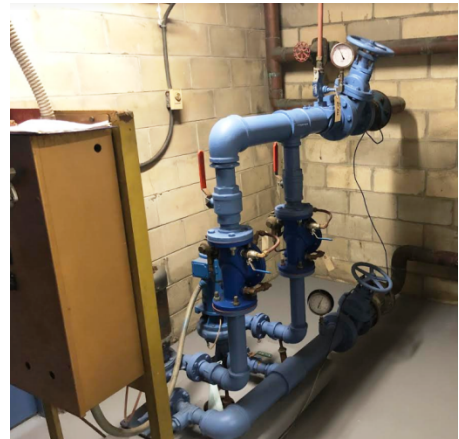
Domestic Water Pump
