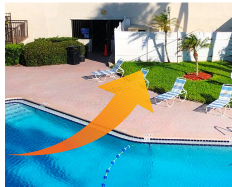
Spa pump, filters & heater are behind the white fence
