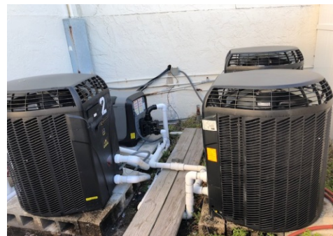
Spa heater is on the right background
