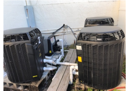
Pool Heaters are the 2 on the left and one at right foreground
