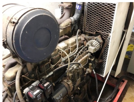
Emergency Diesel Engine
