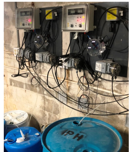
Metering pumps at top of photo. Hypochlorite Sol'n lower left container
