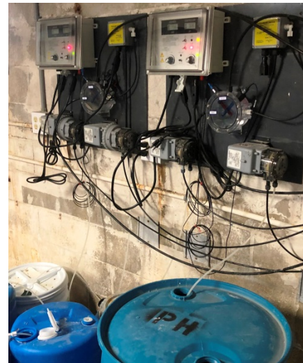
Metering pumps at top of photo. Hypochlorite Sol'n is in bottom left container
